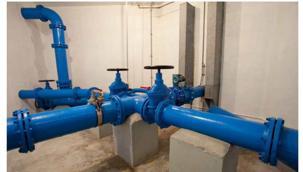
Armature v vodohranu
